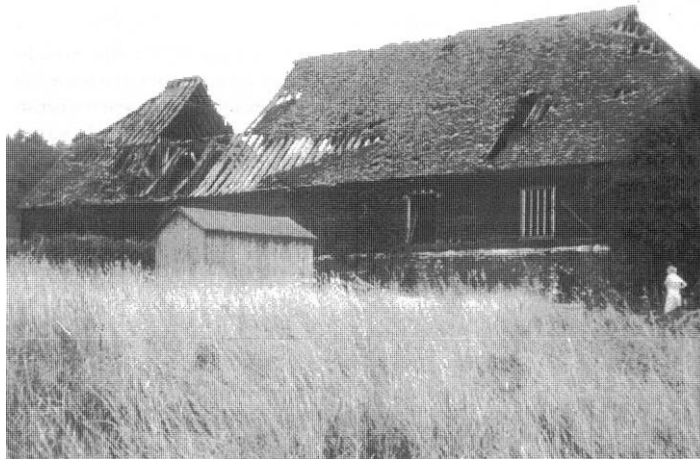
Fig. 16 Croxley Great Barn just before restoration in 1973-5 Photograph courtesy of Three Rivers Museum Trust
